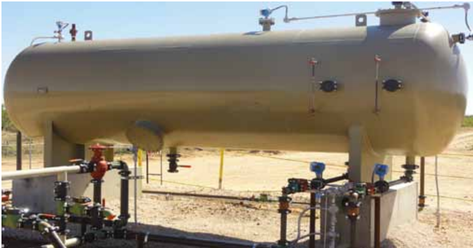
Figure 1: In a separation vessel, oil and water separate, with oil moving to the top and water to the bottom. Capacitance level switches are used to detect the oil/water interface.
