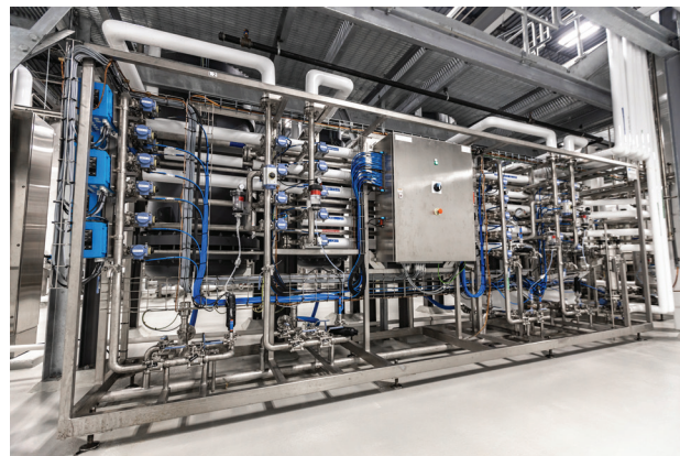
Pre-designed skids help optimize each step of the process
