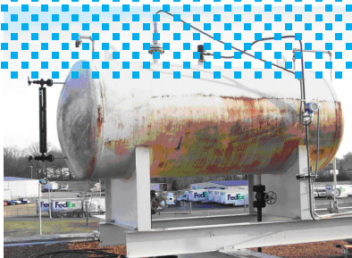
Heating oil storage/expansion vessel mounted on roof
