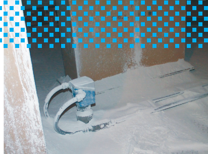
Levelflex installed in lime bin
