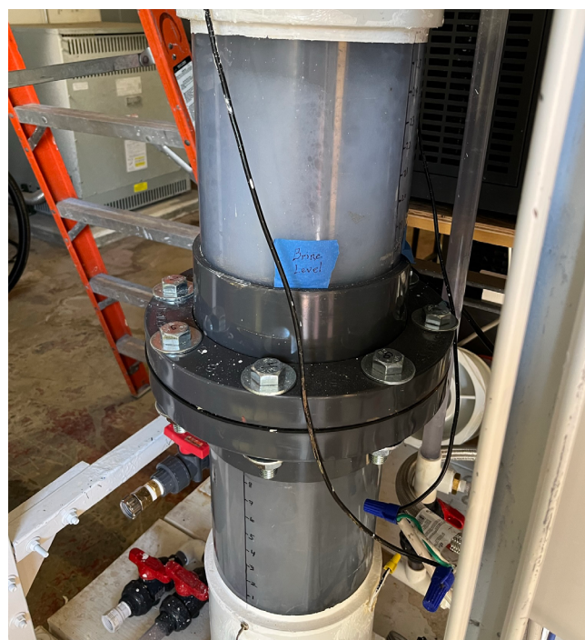
VAED system distilling 110,000+ mg/L TDS concentrate at 122 °F.
