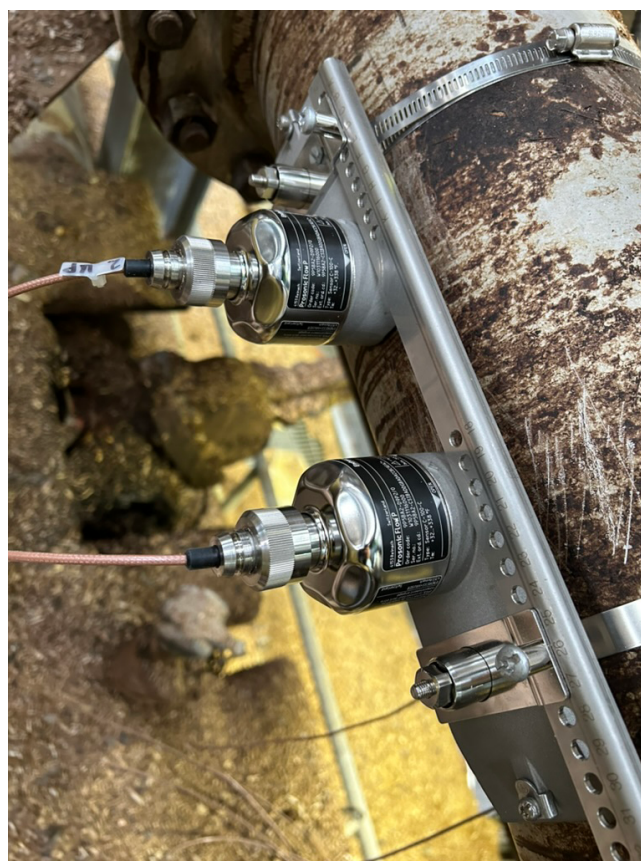
Using the flowmeter's clamp-on method helped ensure the company did not encounter lock-out, depressurization or even shutdown.
