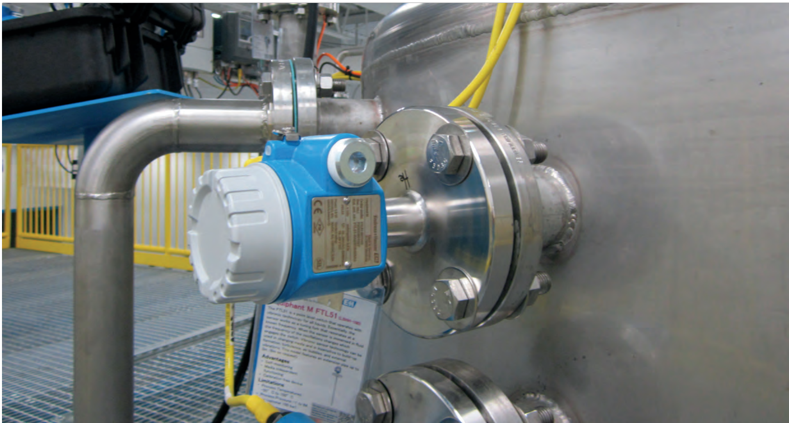
Typical level switch, installed near top of a tank to detect possible overfill conditions. To perform a full proof test often requires removing level switch.
