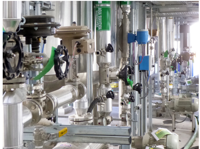
Figure 1: A wide variety of instrument technologies, standards, installation conditions, and operating needs can make it tough for industrial facilities to keep up on calibration needs.
